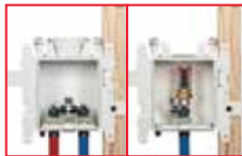
TWO VALVE BOX + ONE VALVE BOX
